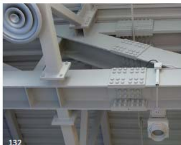
132 Varying approaches to bolting are used to achieve the splicing of the I sections and the joining of the SHS members to the truss.
