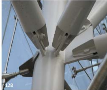
128 Tubular members can be connected using very inventive means. This combination of plates allows for constructability, minimal on site welding and enhanced interest in appearance.
