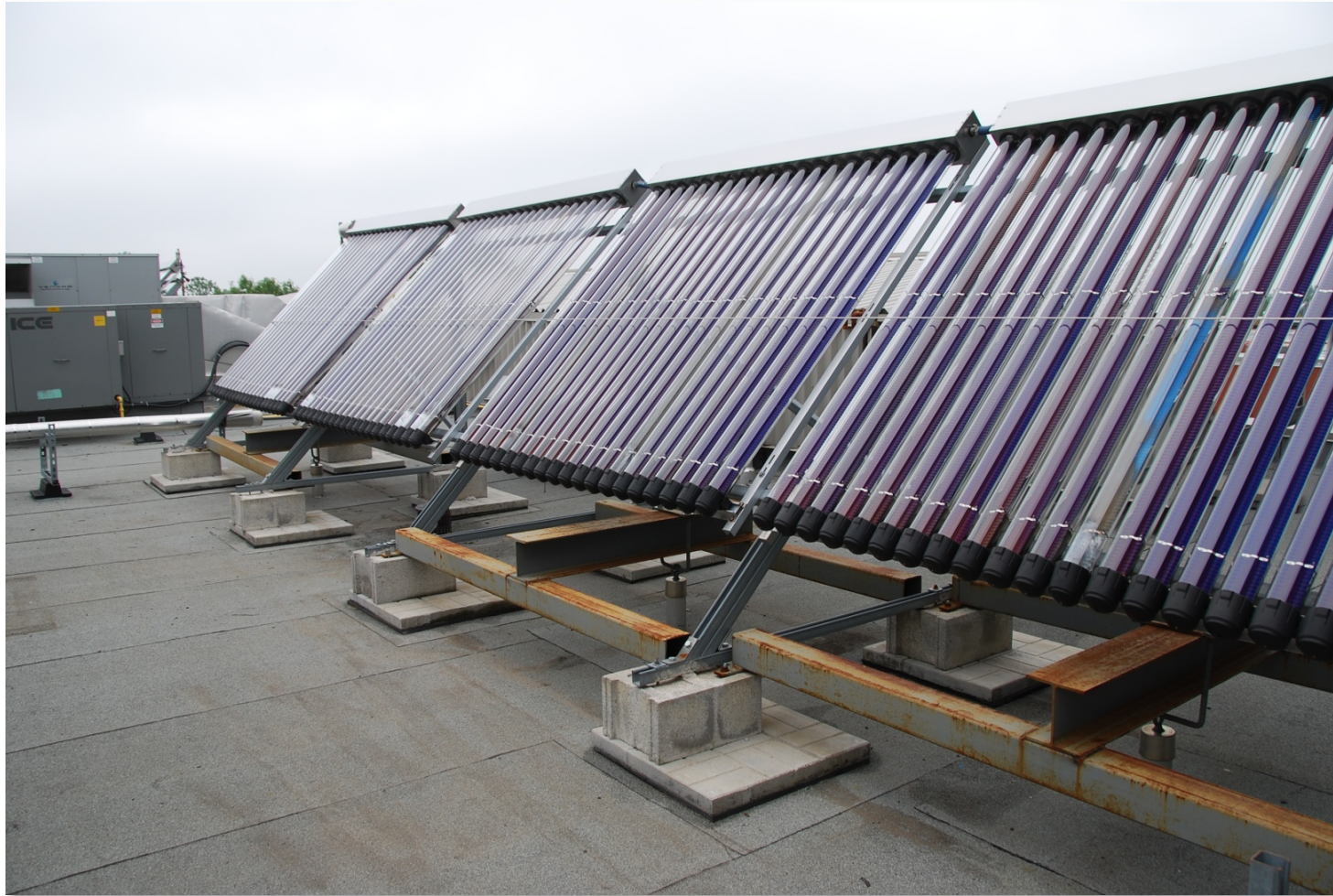
Evacuated tube system at Benny Farm Housing in Montreal.
