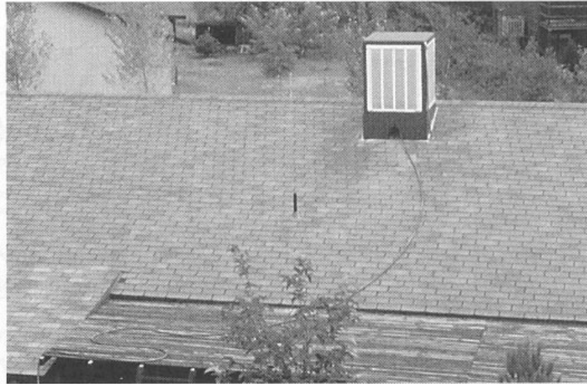
Figure 10.11b Evaporative coolers are widely used in hot and dry regions. This is an example of a direct evaporative cooler on the roof of a house.
