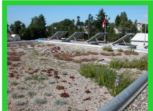
Green roof at White Rock Operations Center, White Rock, B.C.
