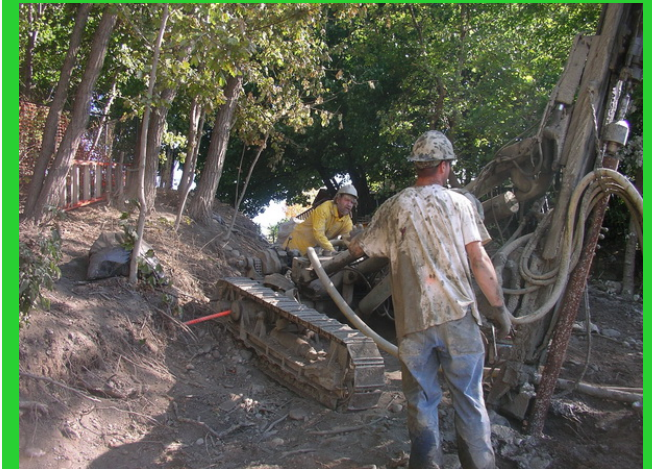
Difficult foundations for a tree, sloped site for the Grand House Student Cooperative in Cambridge, Ontario, Canada
