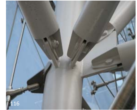
116 Tubular members can be connected using very inventive means. This combination of plates allows for constructability, minimal on site welding and enhanced interest in appearance.
