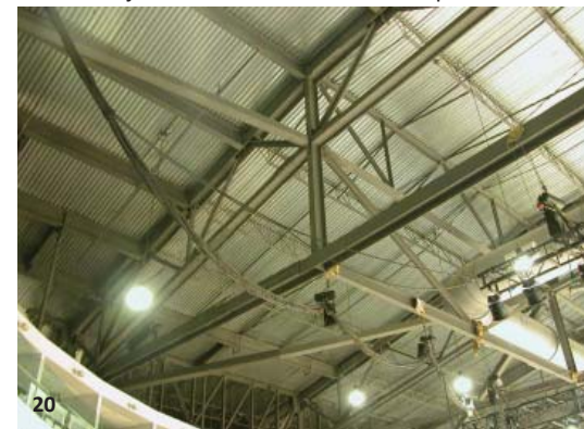
Ricoh Centre, Toronto, ON: Although the trusses that span the arena proper in the Ricoh Centre are somewhat closer to view, they fall into AESS 1 given their more roughly detailed design style as well as the less refined nature of the space. (low cost premium through the use of standard sections and connections that are removed from view)
