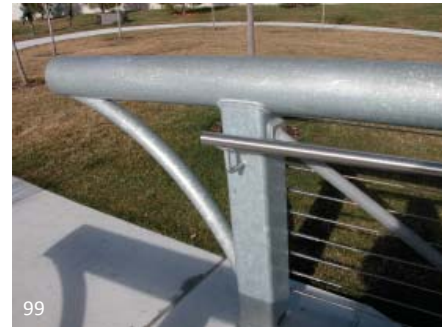
Seal welds have been used to connect the various components of this exterior galvanized steel feature railing. There is a large opening at the base of the square HSS post to allow any water that may enter the railing an opportunity to drain.
