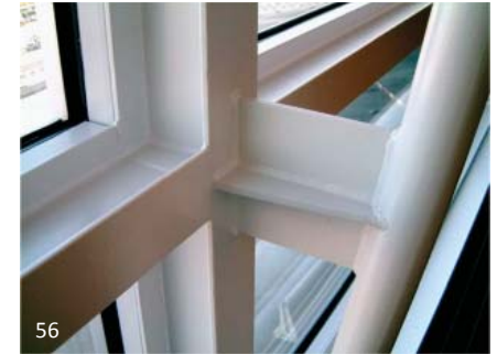
Fig. 2.4B Welds are plainly visible but of good, uniform quality so complementary to the structure.
