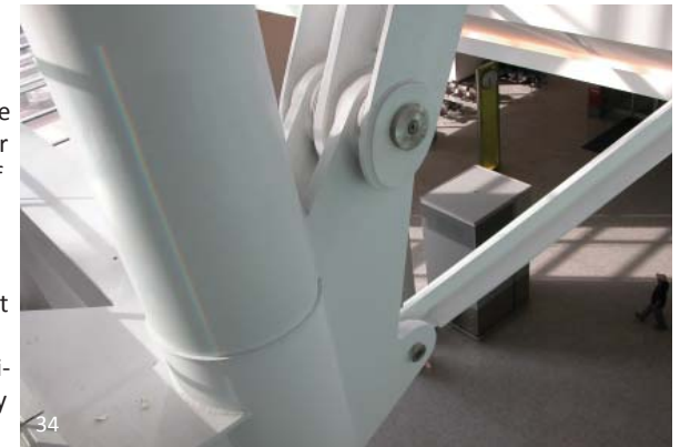
34 Pearson International Airport in Toronto uses a combination of AESS 4 for the columns and supports that are visible in the pedestrian areas, and Custom for the “wishbones” that form the supports for the roof trusses. The supports make use of more standardized shapes where the “wishbones” require significantly more effort on the part of the fabricator in the creation of specialty sections from plate steel.
