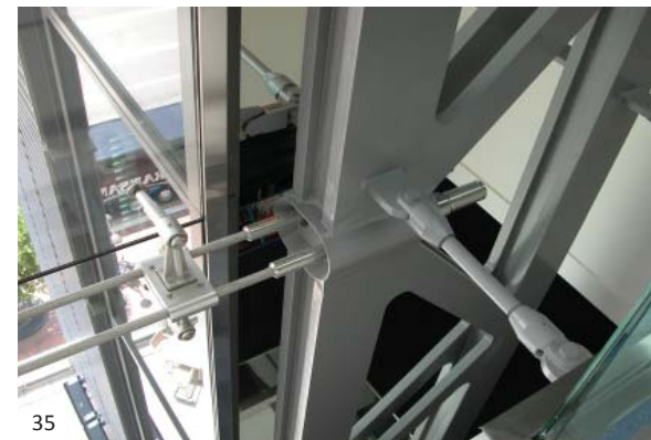
35 The Newseum in Washington, D.C. by Polshek Partnership uses a combination of AESS 4 quality steel with some custom specialty elements in this inventive support system that forms the support and wind bracing for a large mullionless glazed wall at the front of the building. Stainless steel brackets hook on to parallel tension supports that are braced on either side of the façade by these vertical trusses that are fabricated from parallel sections of plate steel.
