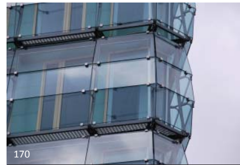
170 The steel supports for this double façade envelope use a system of clips to support the extra layer of glass. This alleviates issues of drilling of the glass and allows for better accommodation of differential movement between the systems.
