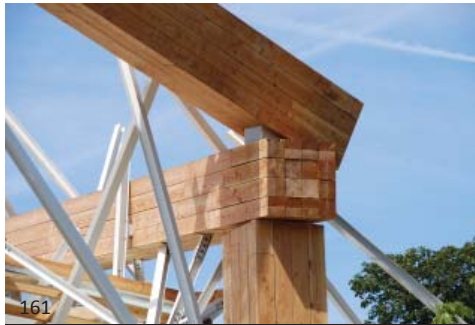
161 The heavy timber on this scupltural project is really "for show" as the main support system is all steel and the large square wood sections are used only to bulk out the form and provide a contrast with the steel used to support the glass.
