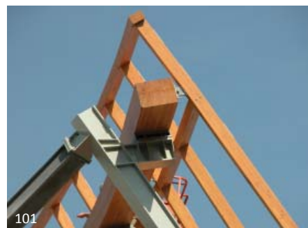
Here galvanized steel members are mixed with zinc painted grey steel. It was decided not to galvanize some of the members due to the chance of deformation in the hot zinc bath and potential stress release of the welds.
