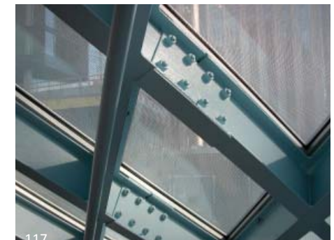
117 This building uses extensive diagrids formed with W sections. These are very simply attached using splice plates on both sides of the flange.
