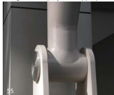
Fig. 2.4A The grinding of these welds incurs a cost premium but is necessary for the seamless look of the connection. This is not universally necessary, especially considering the viewing distance of AESS 2 elements. This treatment should be saved for AESS 4 Characteristic 4.3 Surfaces filled and sanded, where the elements are in close viewing range and sometimes able to be touched.
