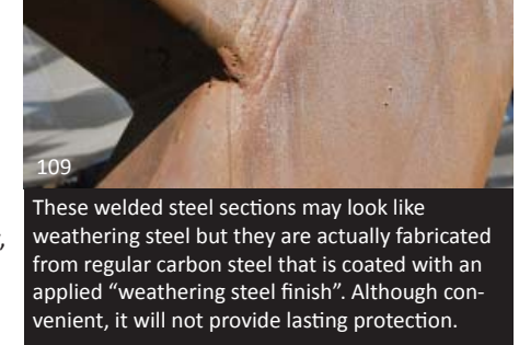
109 These welded steel sections may look like weathering steel but they are actually fabricated from regular carbon steel that is coated with an applied “weathering steel finish”. Although convenient, it will not provide lasting protection.
