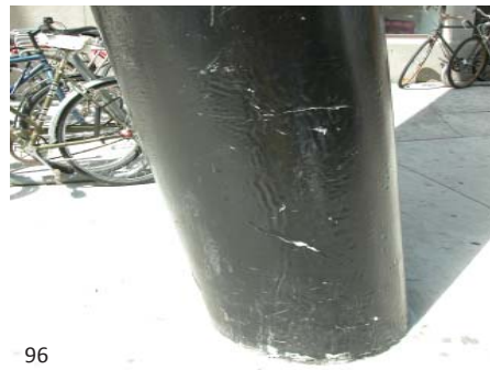
96 This thick intumescent coating is constantly being repaired due to its high traffic location as well as repeated incidences of graffiti removal. The colour matching on some of the supports is more difficult to achieve.
