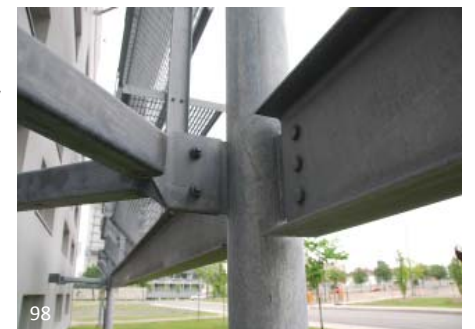
98 As can be seen in this galvanized exposed steel exterior shading system, a variety of finishes can be seen on the different hot dip galvanized members. This is to be expected in this sort of application.
