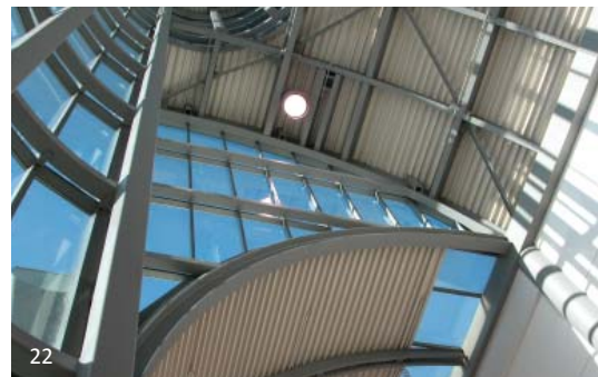
National Trade Centre, Toronto, ON: The project makes use of relatively standard steel sections, but the design and fabrication employs a higher standard in terms of arrangement and detailing. There is some section bending required which increases fabrication costs and can impact detailing. Much of the structure is still located in excess of 6 metres above view.
