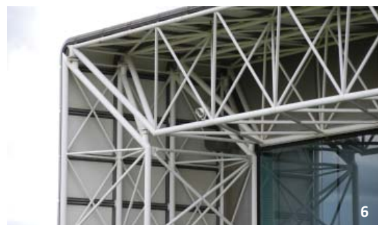
The Sainsbury Centre for the Performing Arts was designed and constructed by Norman Foster in 1977. The British High Tech movement brought exposed structural steel to the forefront of design, and with it an array of issues that had not been part of architectural discourse for more than a century. The project used round HSS members and a structure that was expressed on the exterior and interior of the building.
