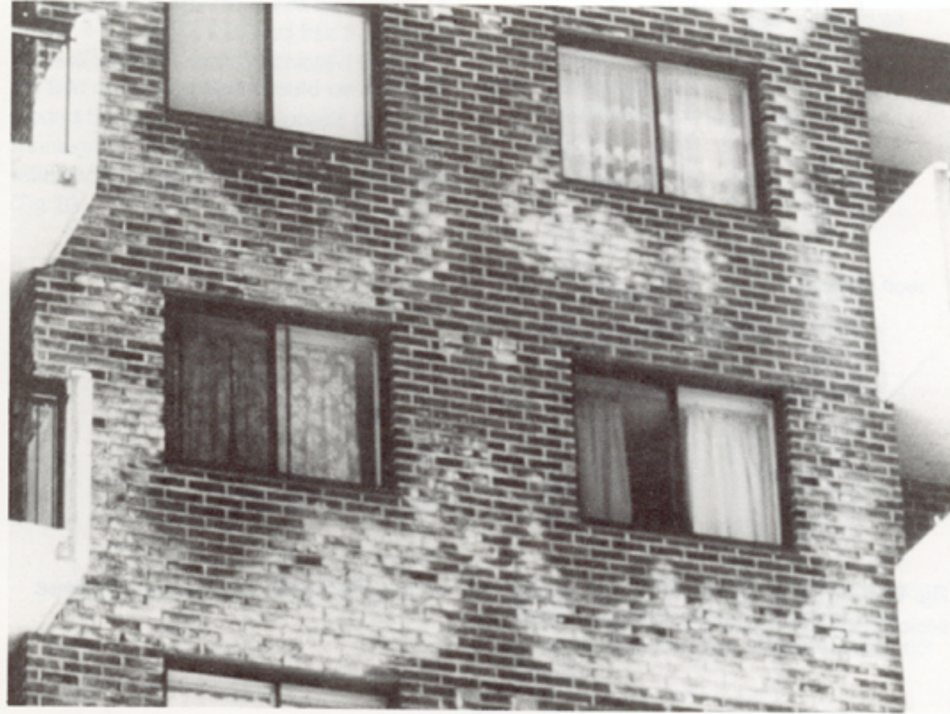
Fig. 16 An example of extensive wetness and efflorescence
