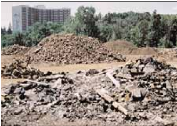
Demolition materials separated for recycling and reuse at the Spencer Creek Village Project in Dundas, Ont. @ http://www.cmhc-schl.gc.ca/rd-dr/en/hr-trs/e_dunda1.htm
