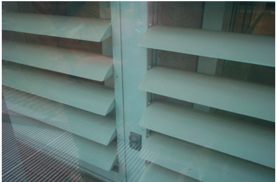
It can be seen that the louvers are fixed in a horizontal position, painted white and are very dirty.
