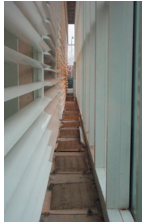
A view inside the cavity showing its clear width to allow for maintenance; the plywood sheets that close off the grille at the base preventing air intake.
