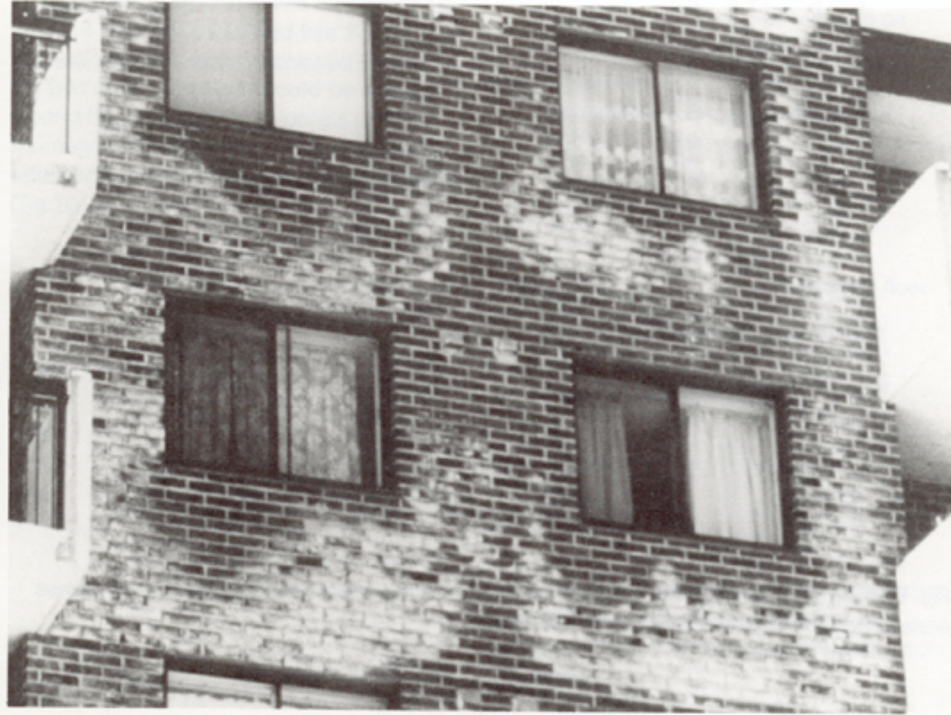
Fig. 16 An example of extensive wetness and efflorescence
