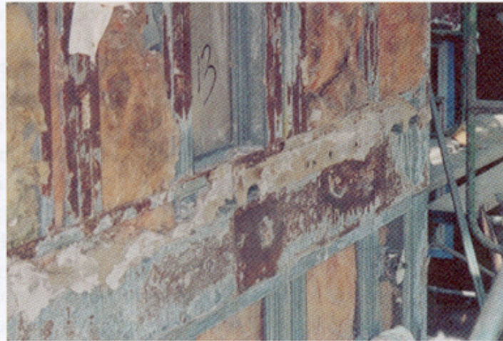
Figure 1: View of severely corroded hot-dip galvanized structural members due to poulitice corrosion from wet building sheathing. Metal loss exceeded 20% of original thickness.
